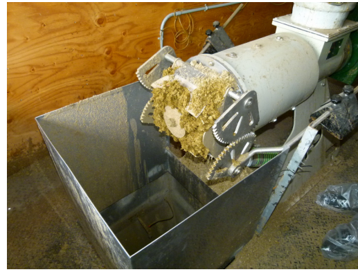
Figure 14 Screw press for separating manure solids
