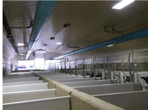
Figure 6 Positive pressure air tube ventilation
